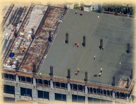
sclarc's new headquarters, which will be called the legacy plaza, gets its roof. (see page 11)
